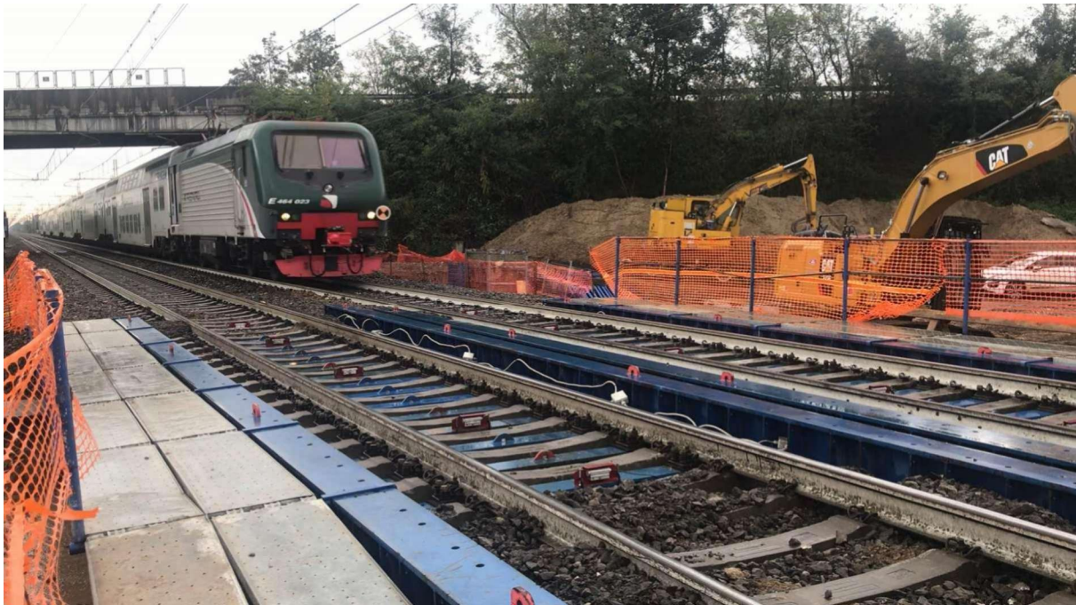
Figure 6 – Petrucco Twist Control Sensors installed on live double track corridor.
