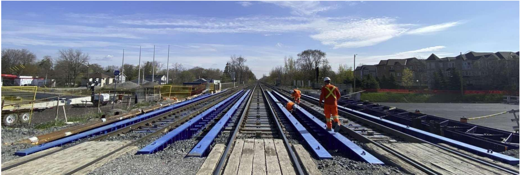
Figure 9 - Flagman & two Petrucco representatives carrying maintenance operations on three active tracks, with both traffics goods and passengers.
