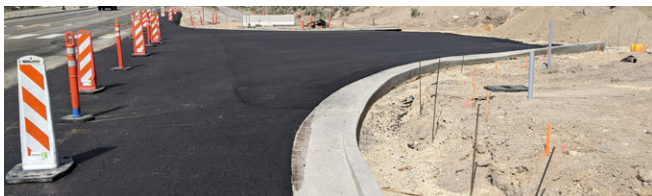
Road construction at Porter Rockwell Boulevard and Freedom Point. Photo credit: Addison Mitton
